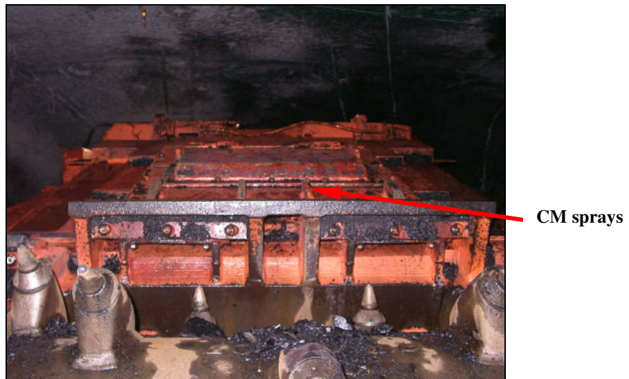
FigureA5: Photographic view of the hood from the front side showing sprays
