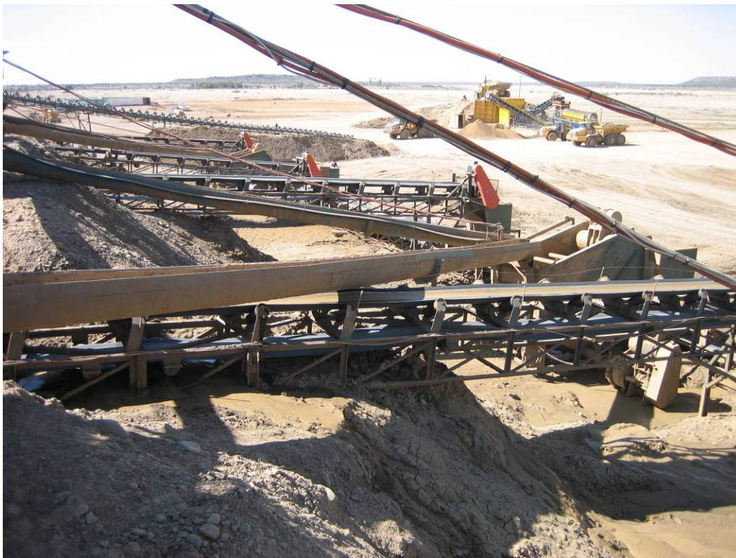
Figure 3.6 Conveyer belts at Rietputs 15.
