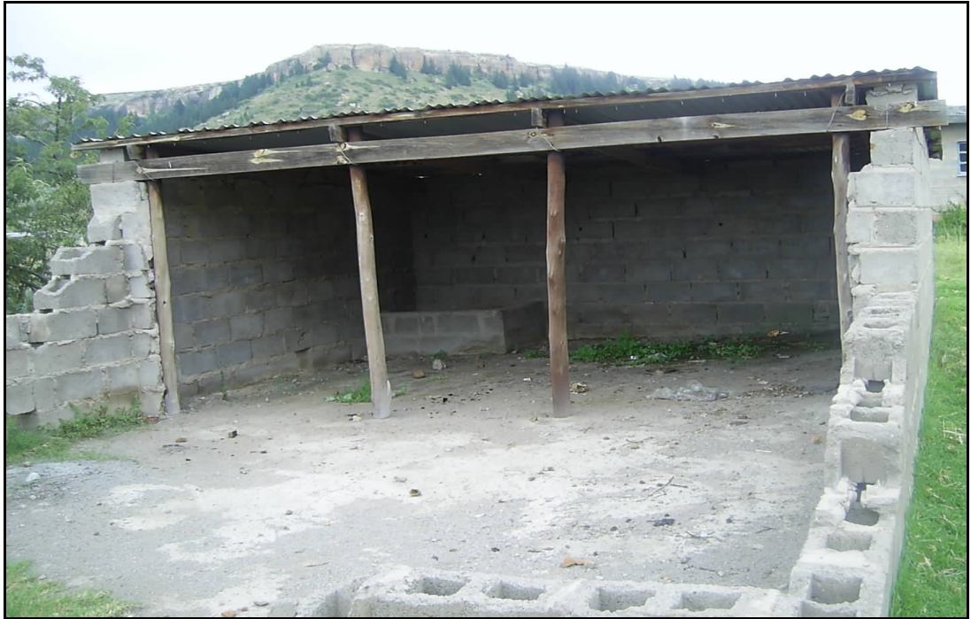
This is what is left of what used to be a shelter for dairy cows.
