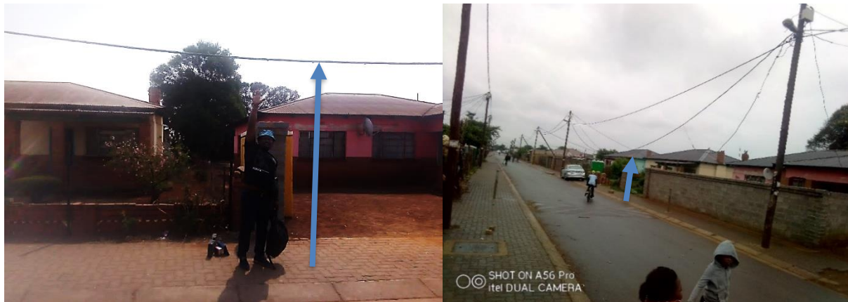
Figure 6.2 Low tension electricity distribution lines in Protea South since 2019, photos taken eight months apart in 2020. Left photo, a resident showing how low the lines drop and right photo showing equally lying lines. Source: Author, 2020
