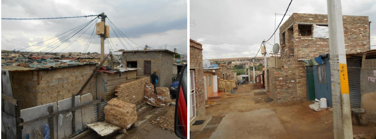
Figure 4.3: Left photo showing electrical pole being incorporated in upcoming brick structure and on the right a storey building under construction is very close to electrical lines. Adopted from Huchzermeyer, 2017
