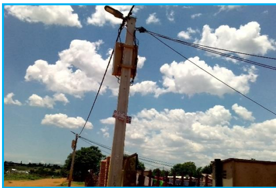
Figure 7.1: A typical electricity pole with meter box and multiple wires going out of meter box in Slovo Park: Source: Author, 2020
