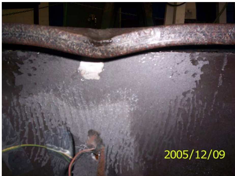
Figure 4.6c – In-plane Local buckling at the point of loading
