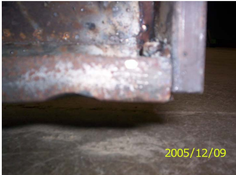
Figure 4.6b – In-plane Local buckling at the support
