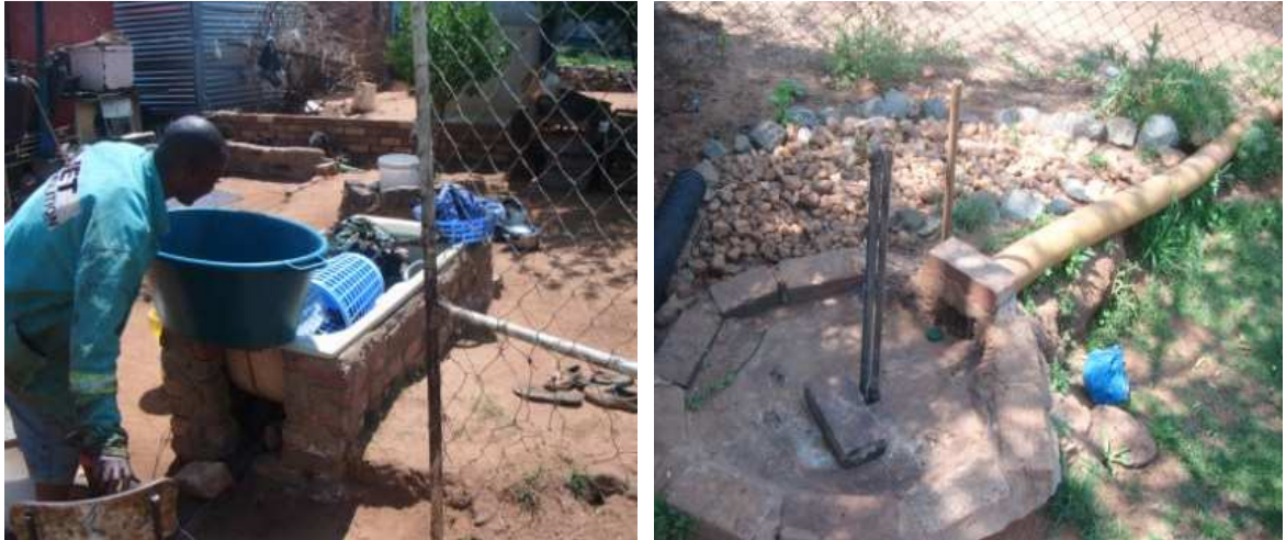
Figure 5.10 Stormwater/Greywater drainage strategies of Elias Motsoaledi residents. Pipe from a old bath tub used for laundry activities (left) and tap stand (right) conveys surface water to gullies on the road.
