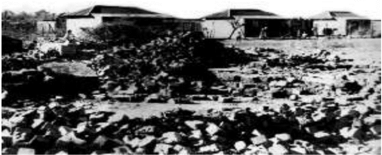
Figure 2.1. Some of the demolished houses in Top Location before the eviction of residents to make way for business activities (Emfuleni Local Municipality. Heritage Book. 14 June 2013).
