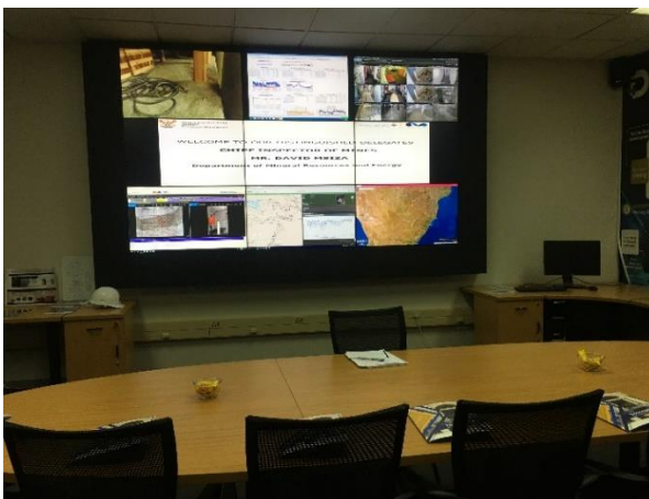
DigiMine control room
