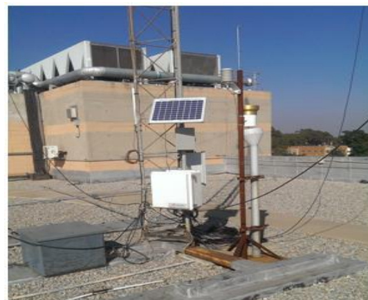
Roof installation of sensors for rain, wind and ambient conditions
