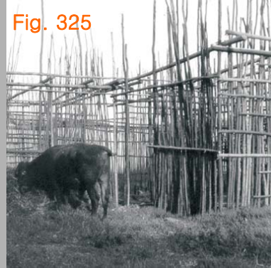
K. Picture to the left shows a traditional structure under construction in East Grahamstown. (fig 325)
