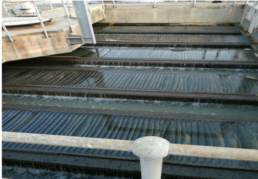
Figure 1.4: Photograph of the sedimentation tank with lamella plates
