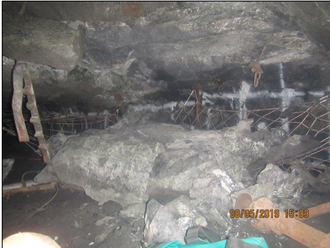
Figure 1-8: Typical rocks which fell with temporary support
