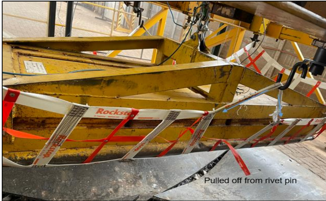
Figure 5-3: Failure mechanism along the two tonnes Rock-stop safety net and 16 mm S-hooks
