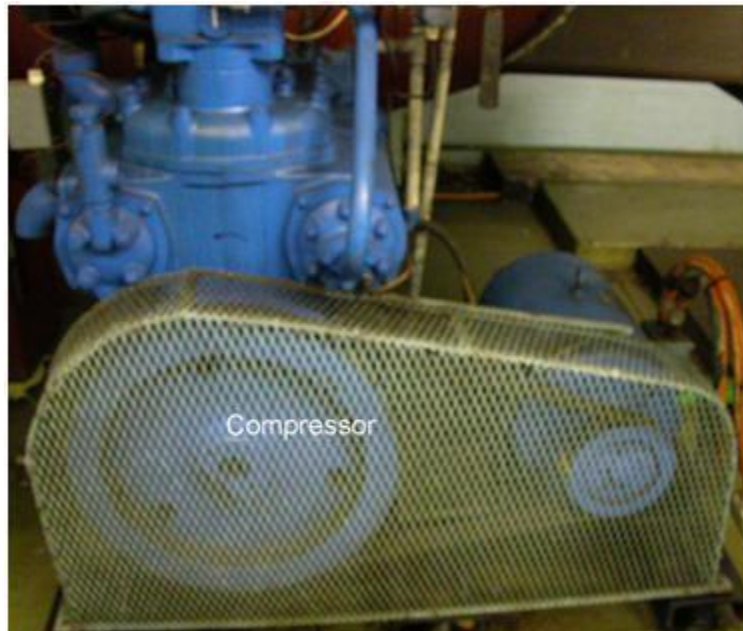
Figure A. 2: Reciprocating compressor
