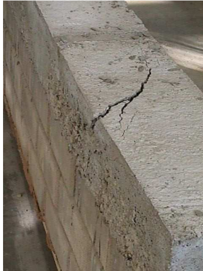
Figure - 5.10: Inclined crack
