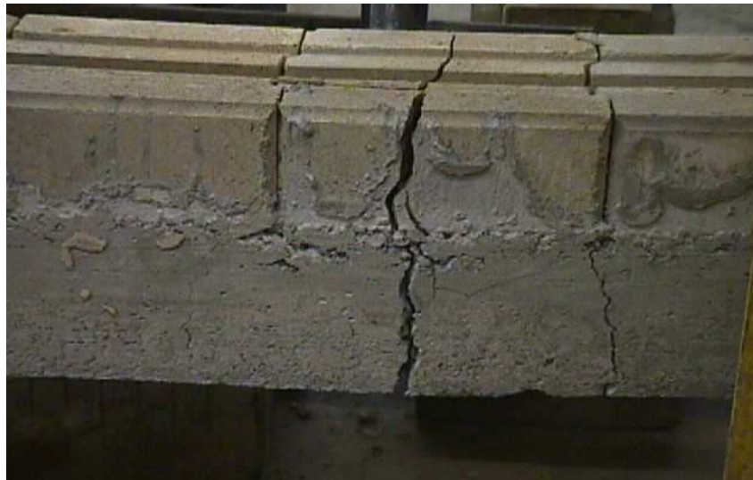
Figure - 5.9: Vertical flexural cracks
