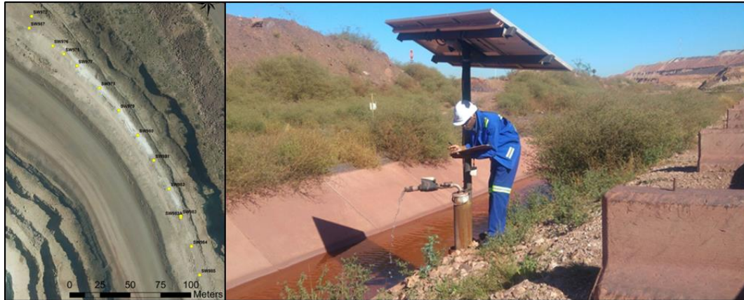
Figure 101 Location of solar powered depressurisation holes with discharge into lined storm water canal.
