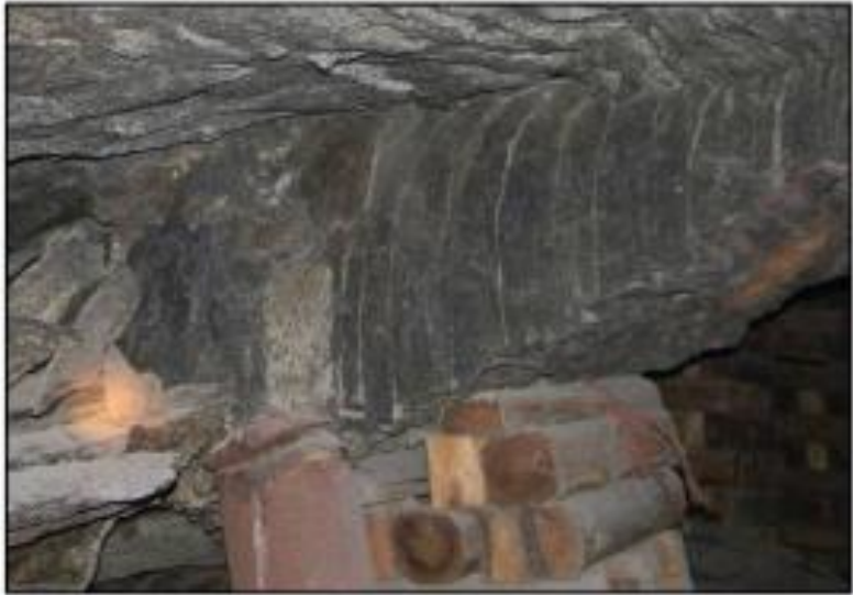
Figure 2-9 Dense, steep dipping and blocky fracturing in Pyroxenite (Mine Health and Safety Council, 2016)
