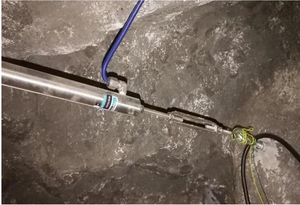
Figure 10: Ground Movement Sensor on tunnel ceiling.
