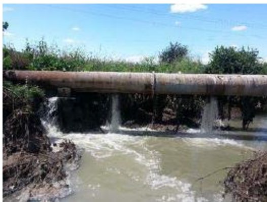
Figure 3: Surcharging Sewer Pipe (Dorner et al, 2014).
