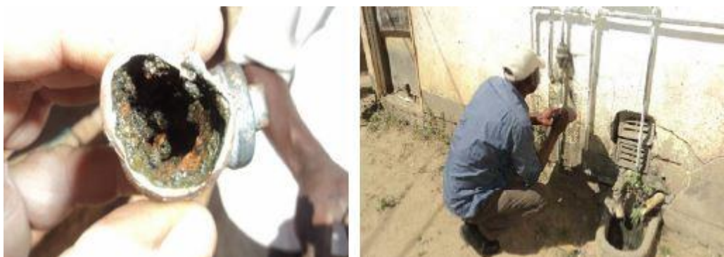
Figure 8: Corroded Household Connections (Dorner et al, 2014).
