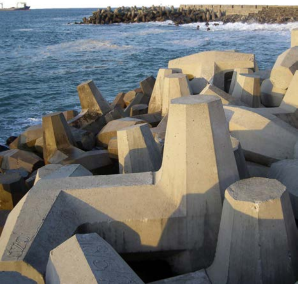
figure 4,13. Dolosse along the Cape Town harbour
