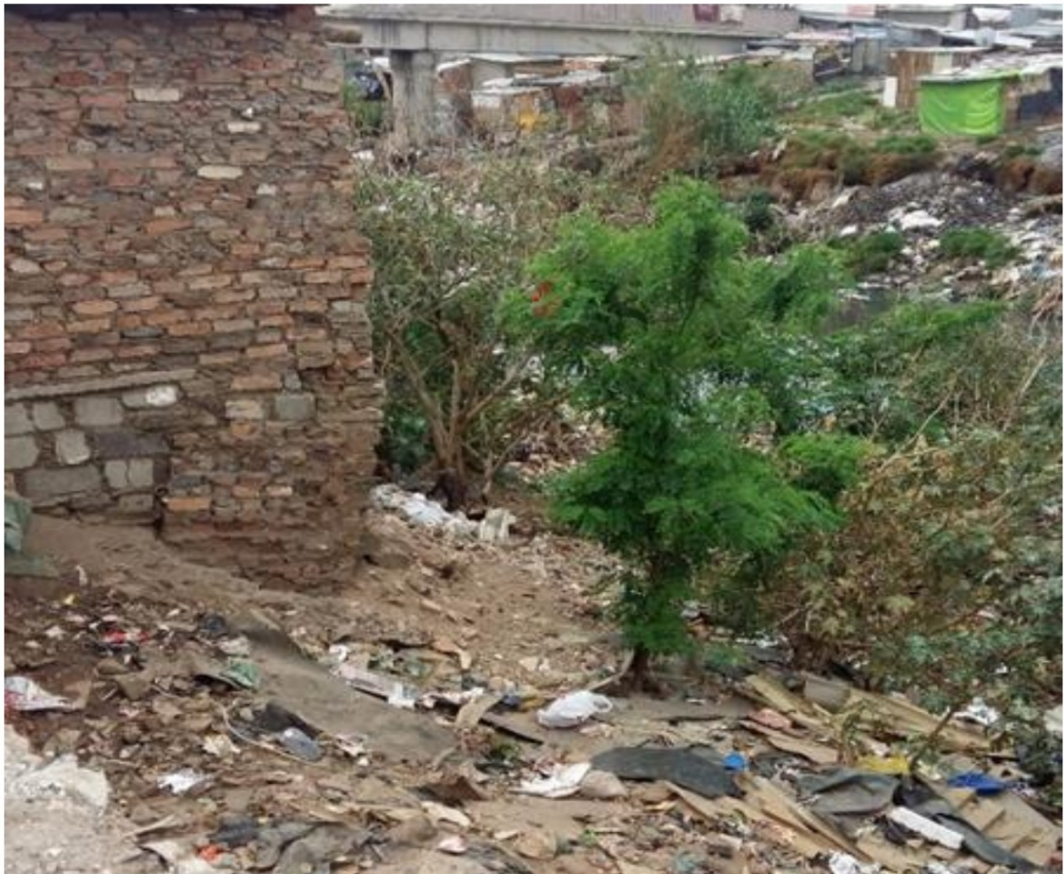
Fig 4.3 The banks of the Jukskei River falling inside. Source: Own (2019)
