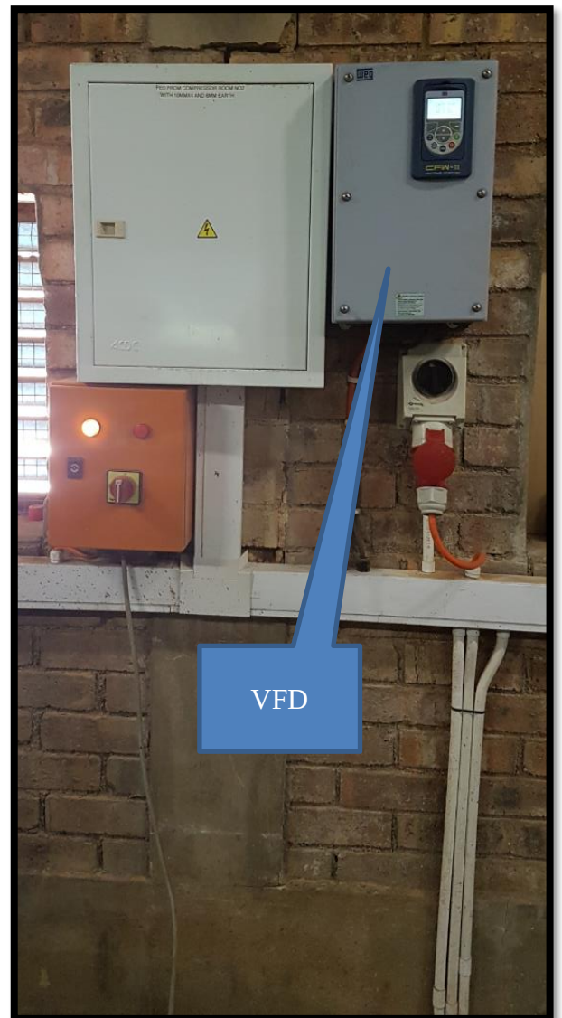
Figure 4-47: VFD used on the test facility.
