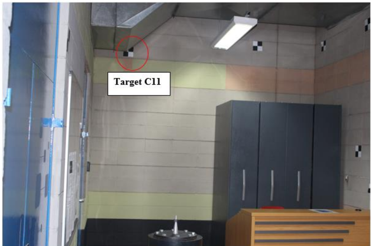
Figure 6.1: Showing Target C11 Being Partially Blocked by the Ventilating Duct
