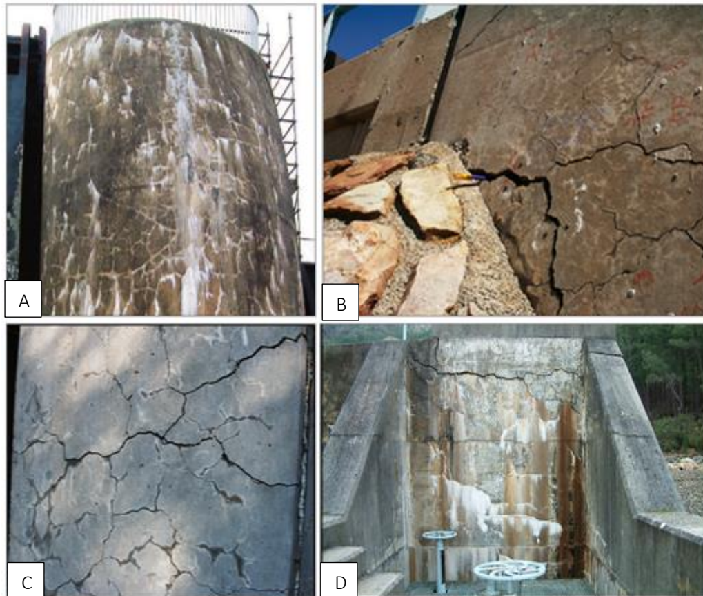
Figure 2.3: A) Concrete structure subjected to ASR showing sizeable cracks and white staining below cracks (efflorescence) (Werner et al. , 2015). B) Cracking (up to 15 mm wide) of the south abutment bridge near Wits Yale/Empire Road entrance, Johannesburg (photo courtesy Y. Ballim). C) Map cracking of the North abutment M1 bridge on Empire Road, Johannesburg, Gauteng (photo courtesy Y. Ballim). D) ASR damaged structure at weir, Western Cape (photo courtesy of Y. Ballim).
