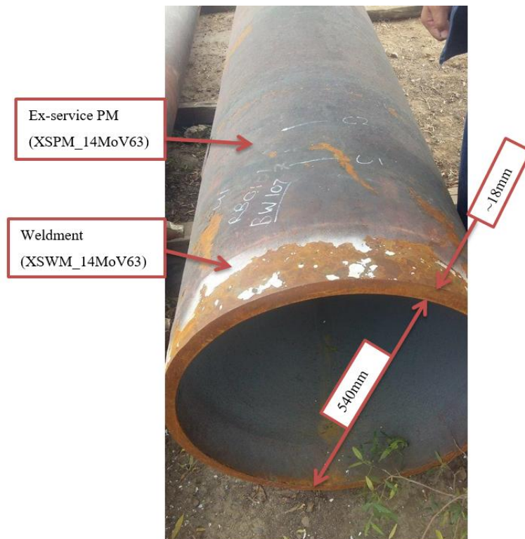
Figure 3.1 Service-exposed 14MoV63 pipe
