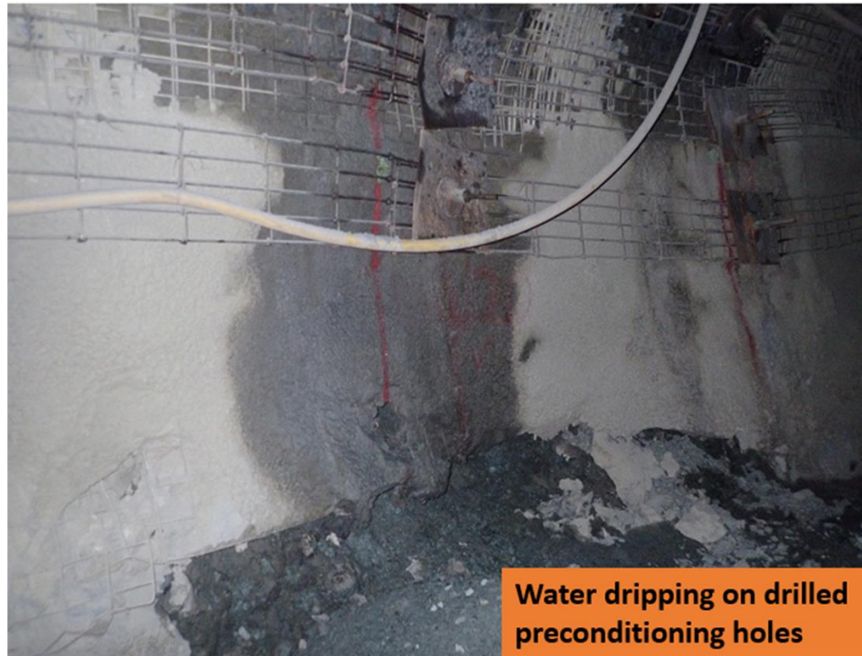
Figure E-1: Presence of water at the weak zone
