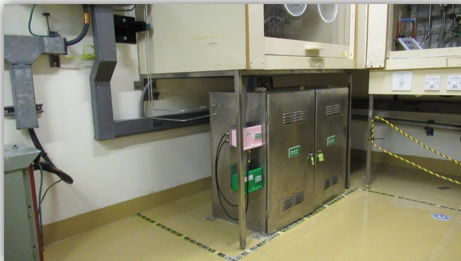
Figure 6.1: Koeberg's zinc injection unit (closed)
