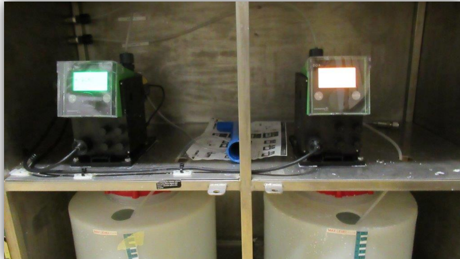
Figure 6.2: Koeberg's zinc injection unit (open)
