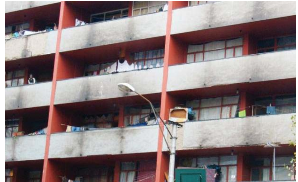
Fig 4.2, San Jose, a "condemned" building in Hillbrow
