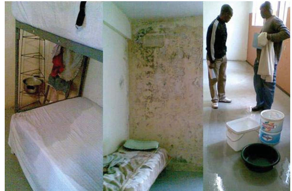
Fig 4.3, San Jose, a "condemned" building in Hillbrow
