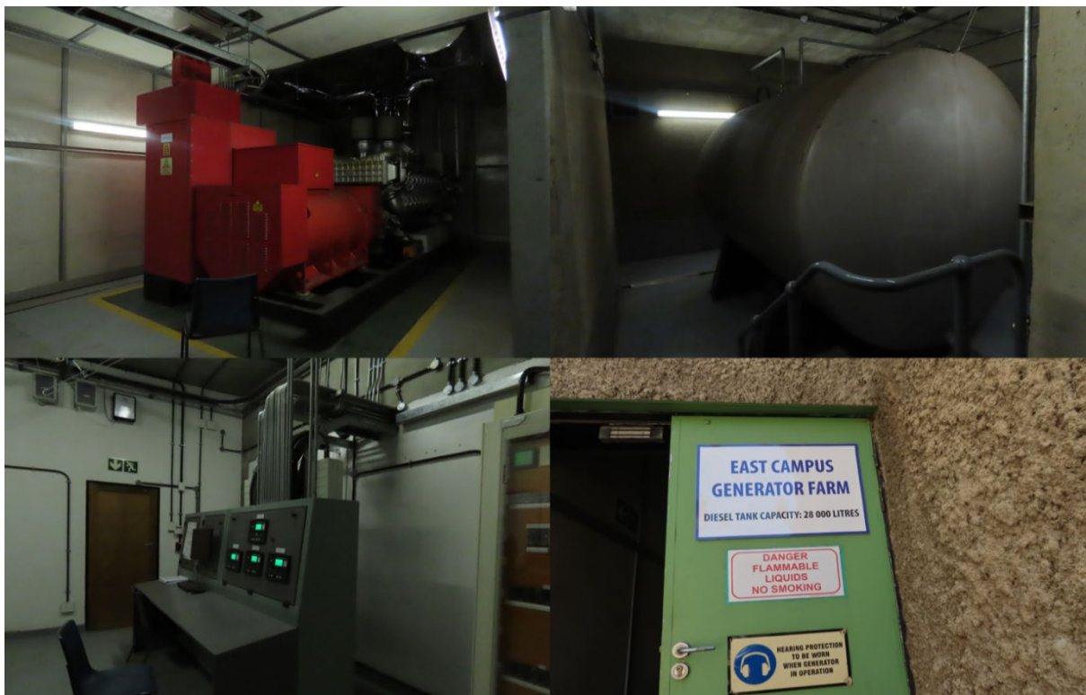
Figure 17: East Campus Generator Farm, 28 000 litres of diesel tank capacity, to power the entire East Campus infrastructure, with 5.5 MVA energy demand (Rodney Matentshi, 2020).
