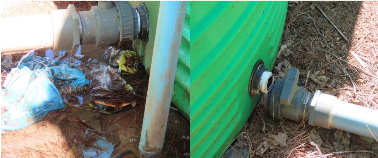
Figure 12: Borehole system at Wits Sturrock Park, west campus, leaking due to lack of water management system and capital funding (Rodney Matentshi, 2020).
