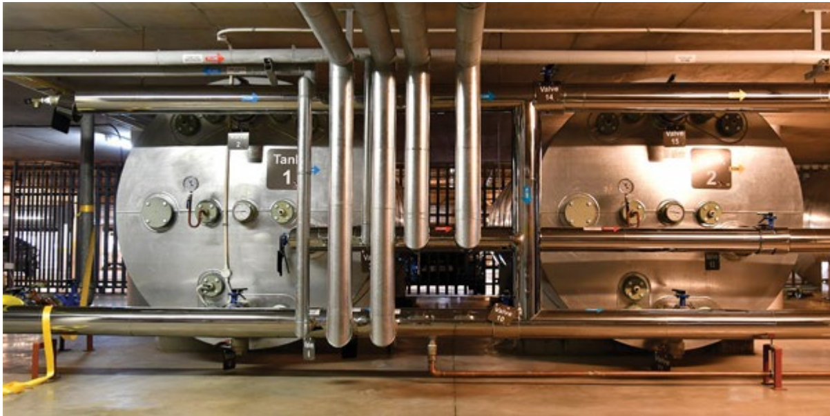
Figure 18: Wits university solar thermal hot water system to meet the demand of hot water of the student residence (Buhle Zuma, 2020).
