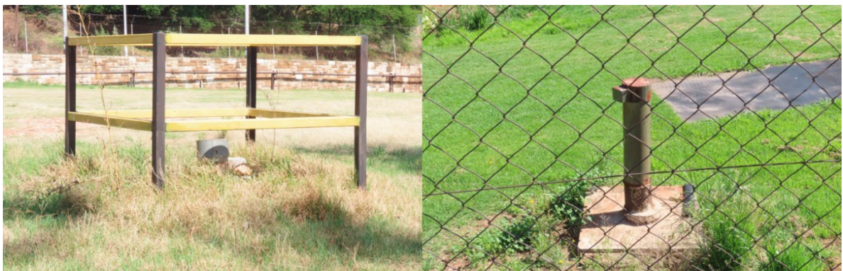
Figure 11: Borehole system at Wits Sturrock Park, west campus, connected to eight of Jojo water tanks storing 80 000 litres for watering Wits Sturrock Park Stadium soccer field (Rodney Matentshi, 2020).
