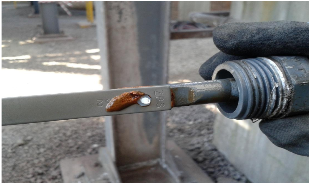
Figure 3-2 Coupon that has been taken out of the return water line, for demonstration
