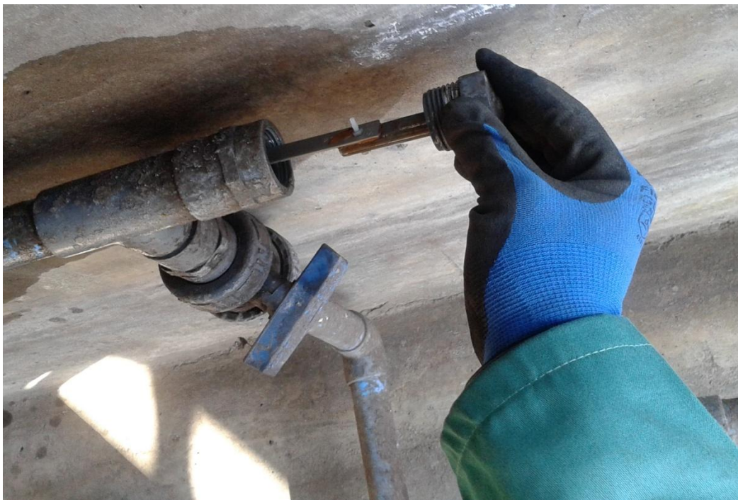
Figure 3-4 Corrosion coupon insertion
