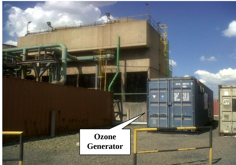
Figure 2-9 Typical ozone generator next to the cooling tower
