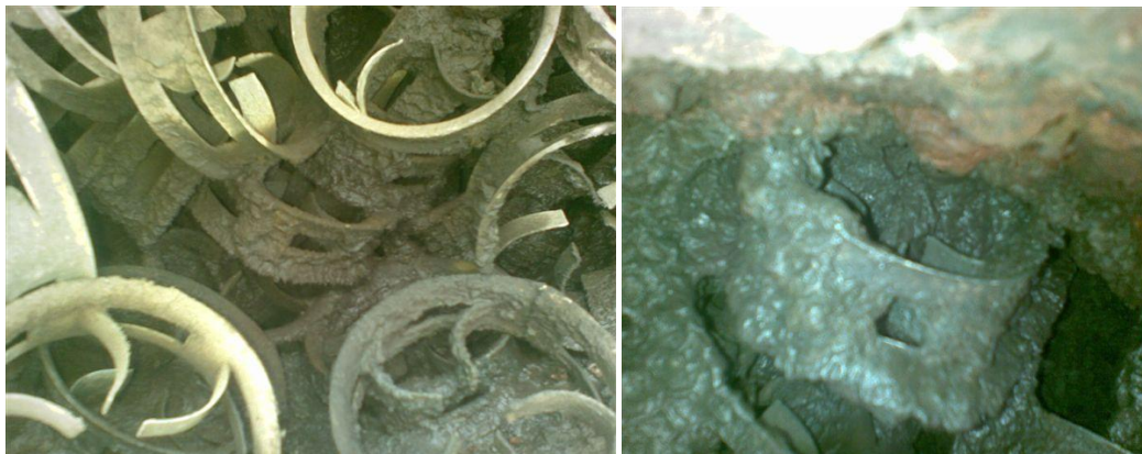
Figure 2-5 Clogged packing inside direct contact after cooler (DCAC) vessel
