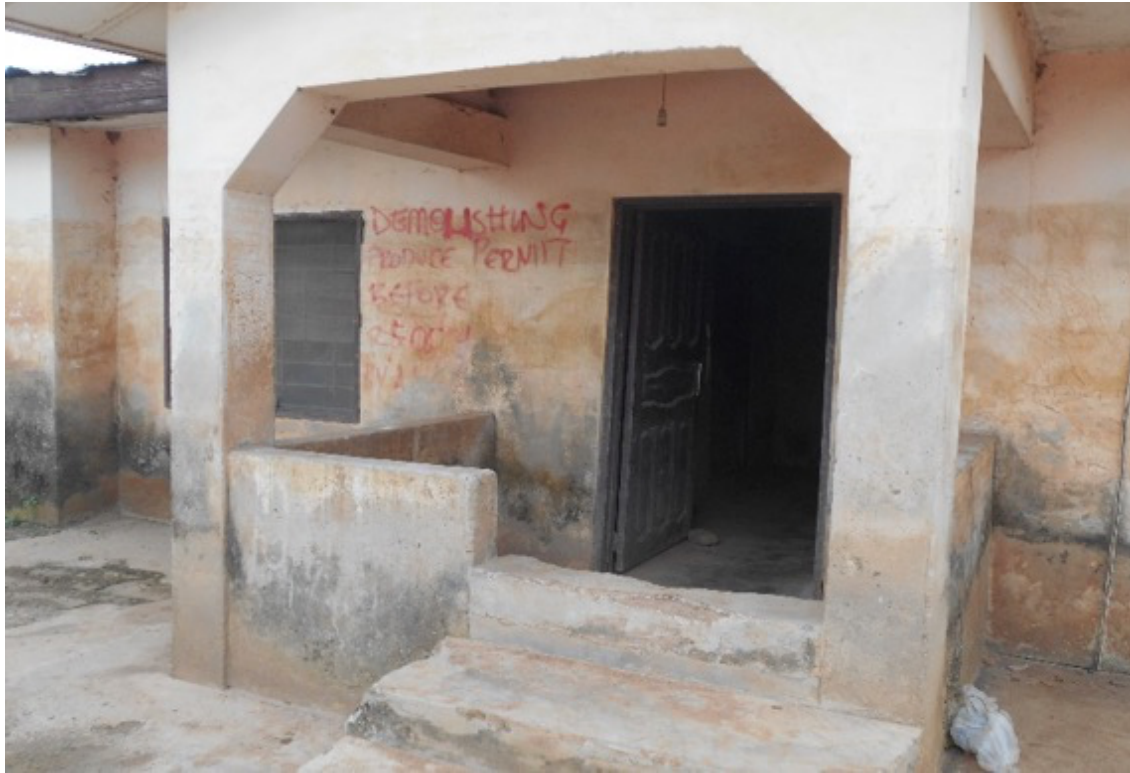
Figure 5.14: Building on an unauthorised plot earmarked for demolition for non-compliance
