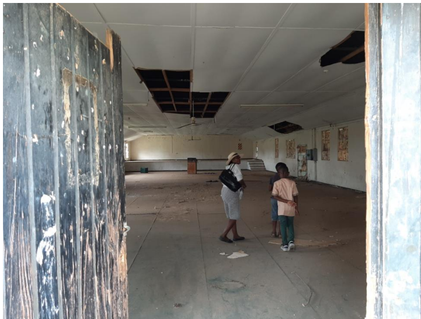
Figure 4: The neglected hall is falling apart. Photo: Author
