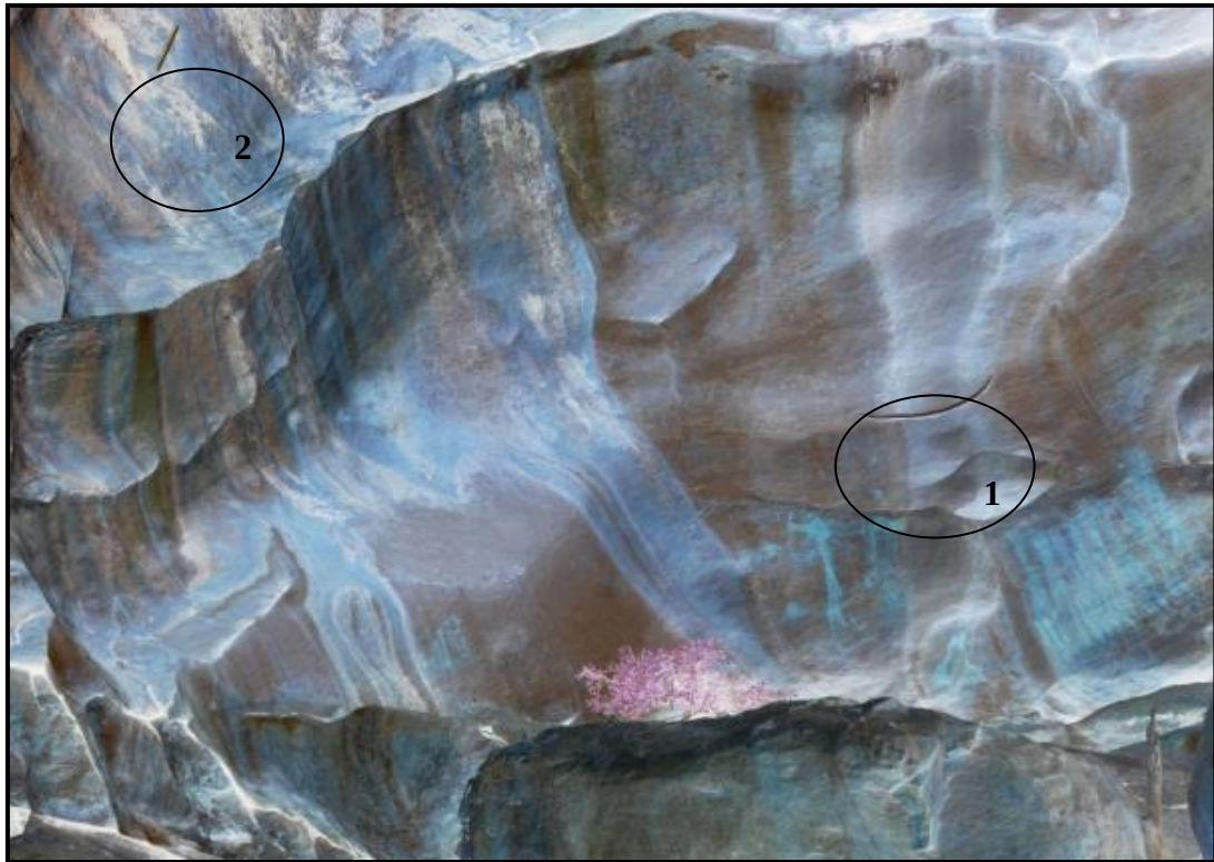
Figure 10: Drip lines interventions at BKS 03
