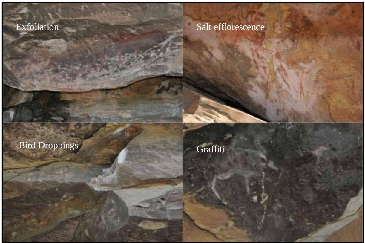
Figure 18: Factors causing deterioration at Main Caves, Drakensberg [Photos by Elijah Katsetse; 2013]
