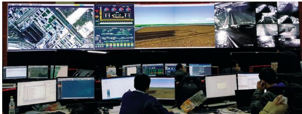
Figure 2.9 Operations monitoring and control center at Jinjie ( Jianguo, 2015 )
