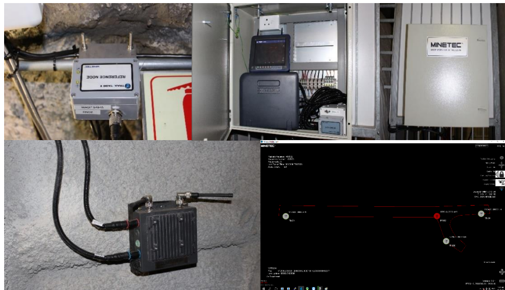
Figure 4.17 Minetec tracking and positioning system Referencing node, control cabinet, data collector/transmitter and real time tracking display (Source: Author)
