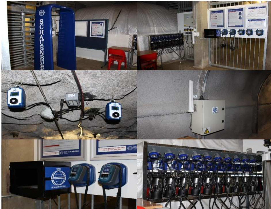
Figure 4.15 Schauenburg's system in the Mockup-mine. Access control, PPE, Gas detection instruments, environmental sensors and S-link for location monitoring (Source: Author)
