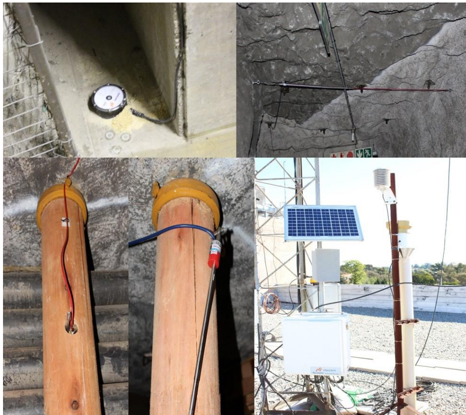
Figure 4.13 Vibra-Tech sensors Seismometer, extensometers and weather station (Source: Author)
