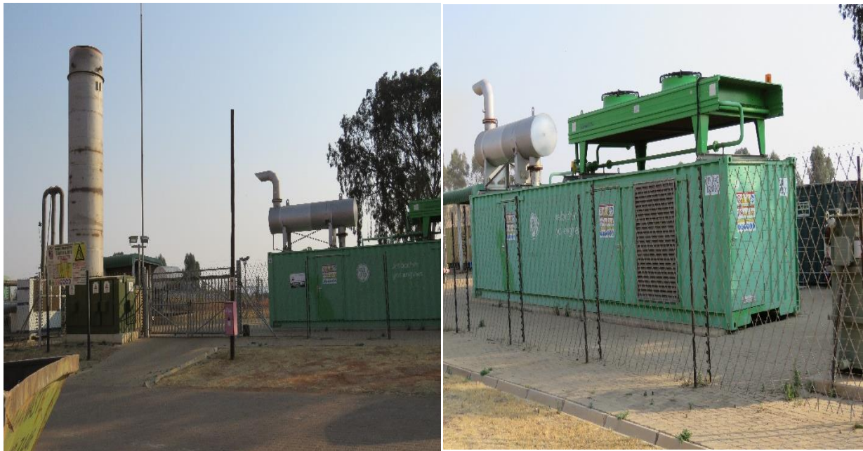
Figure 4.3: 1MW Simmer and Jack Landfill Gas Power Project (Source, Field observation, October, 2019)
