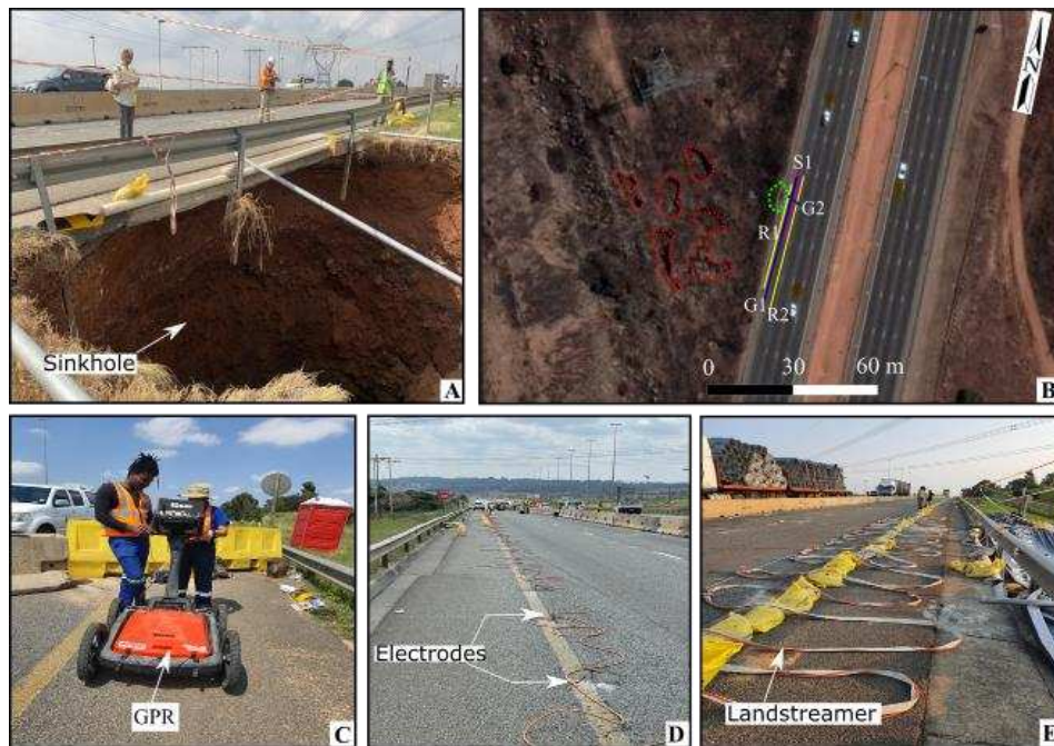
Figure 1: Figure 1a, shows the sinkhole formed along the highway, while figure 1b shows its position (green circle). Sinkholes formed prior to the R21 highway sinkhole are shown in red in Figure 1b. Figure 1c, 1d, and 1e shows the ground penetrating radar, electrical resistivity tomography and seismic land streamer methods, respectively. Photos in Figure 1a, 1c were taken by Musa Manzi.
