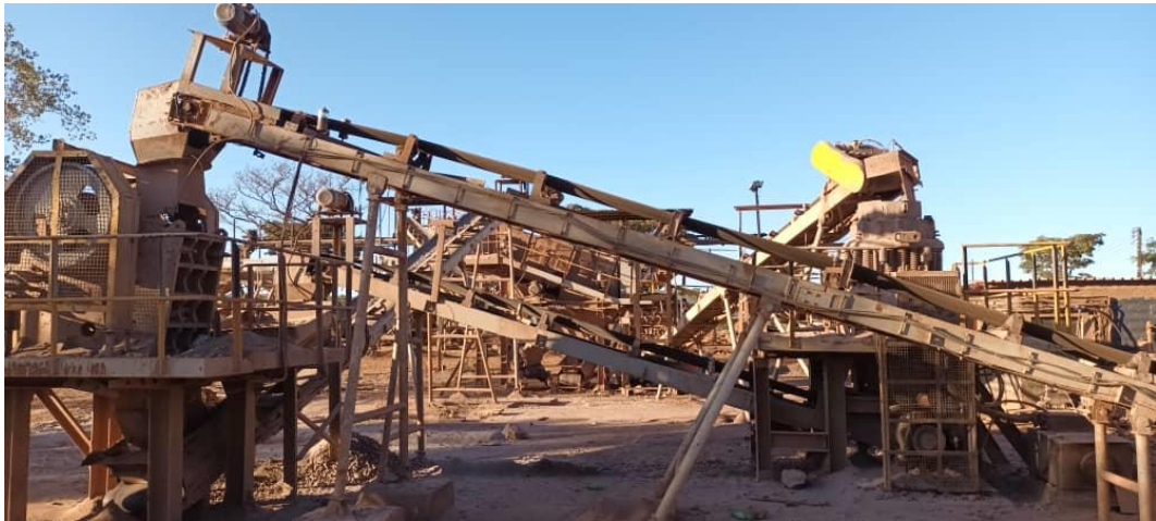
Figure B7 Picture of the PMC crushing section
