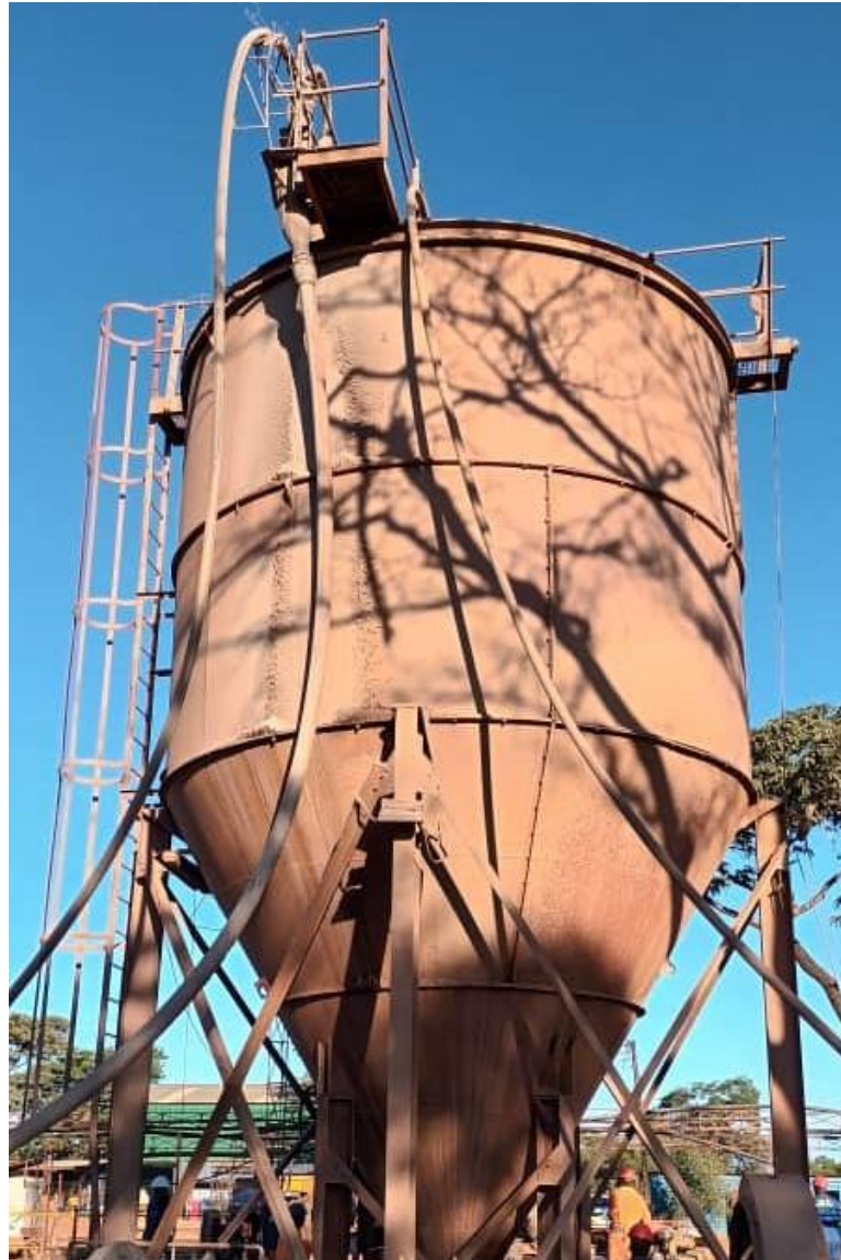
Figure B12 Picture of the holding tank for tailings to the CIL plant
