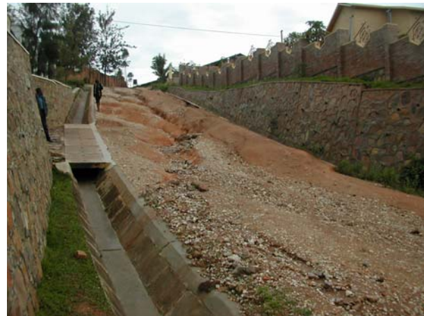
Figure 4.7 Erosion In Kigali Street After Heavy Rain
