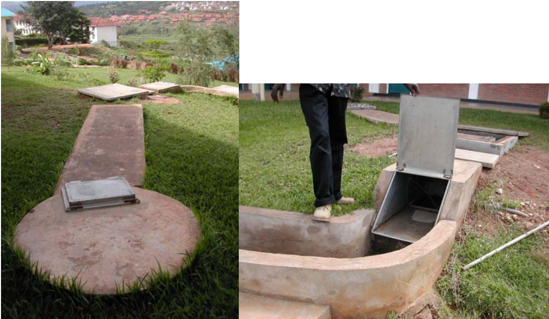
Picture 14. The collection sump leading to the underground tank and the overflow tank and flap to prevent the ingress of insets
