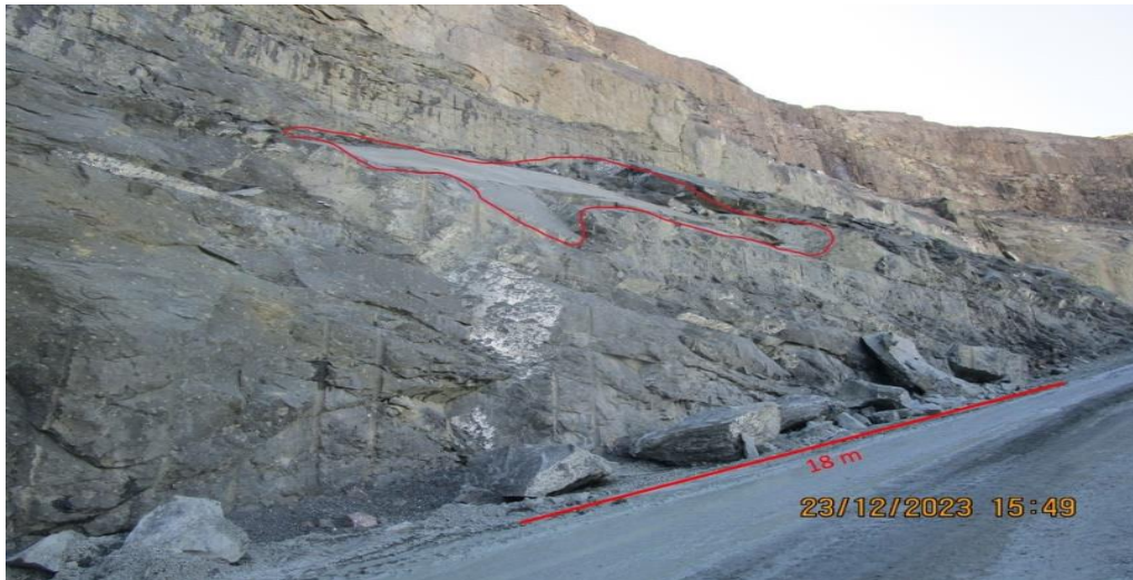
Figure 4-15: An example of high wall crest failure
