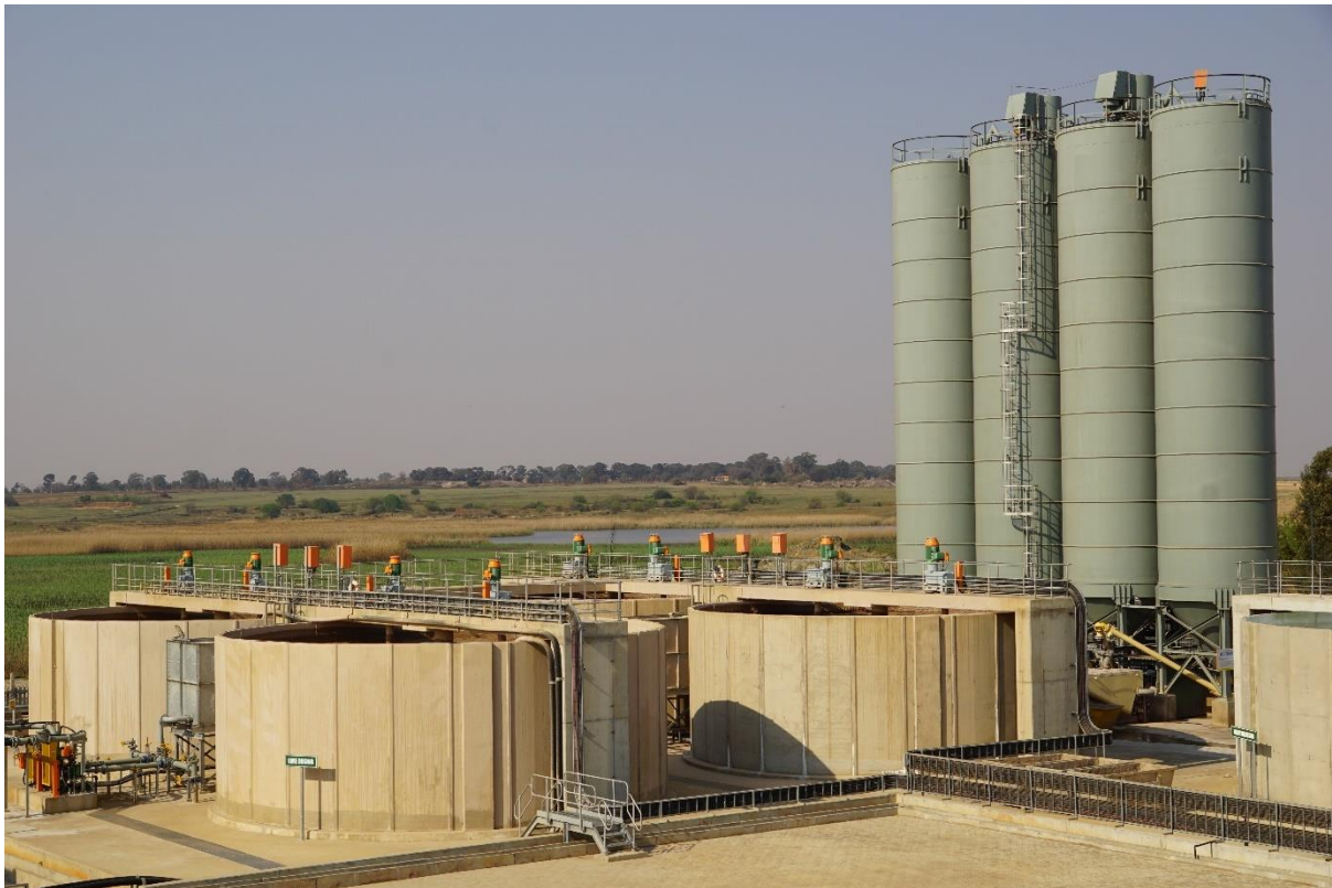
Figure 4: The lime thickener tanks at the new Eastern Basin AMD Treatment Plant, the wetland can be seen behind the treatment plant in the background. Photo taken by Professor C. Curtis in 2017.
