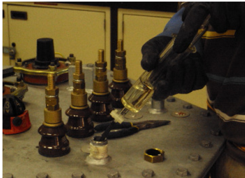
Figure 24: Hexa-transformer oil sampling
