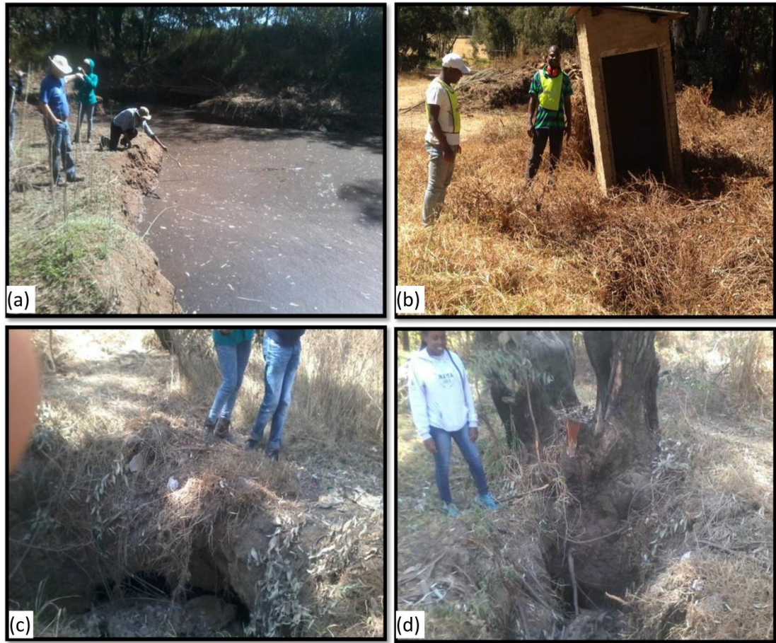
Figure 3.2: Surface evidence of recent subsidence-related events at Benoni area. (a) Water-filled subsidence (b) Abandoned leaning structure caused by subsidence (c) Sinkholes caused by the collapse of the colliery roof into mined-out zone (d) A recently formed sinkhole.
