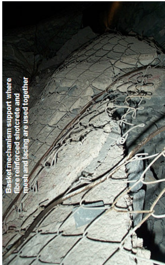
Figure 5.4 Basket mechanism where shotcrete has been applied together with rock bolts; mesh and lacing support (Mponeng Mine Level 116)
