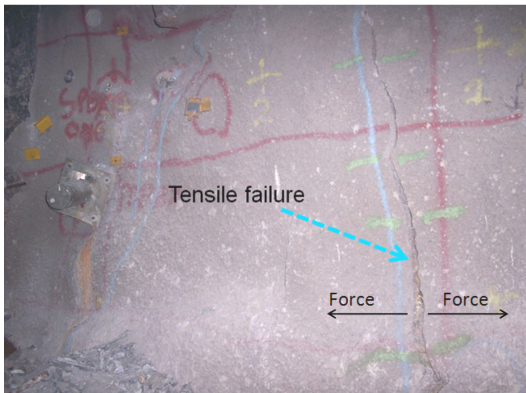
Figure 3.32 Photograph showing tensile failure of shotcrete on Pillar B at South Deep Mine
