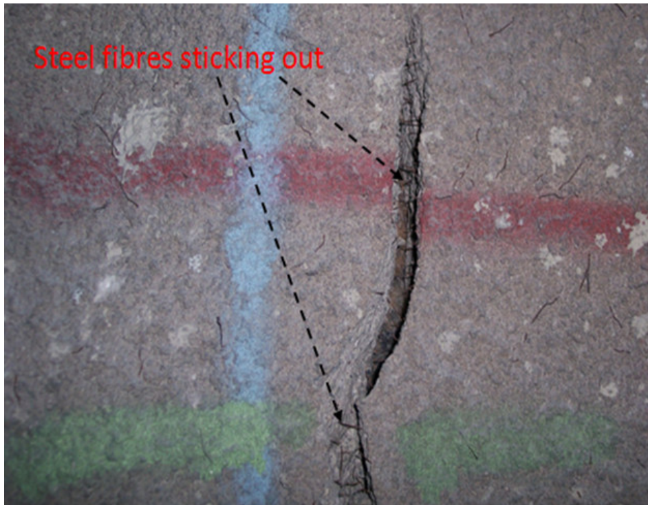
Figure 5.2 Fibres sticking out due to tensile stresses on a shotcrete crack at South Deep Mine
