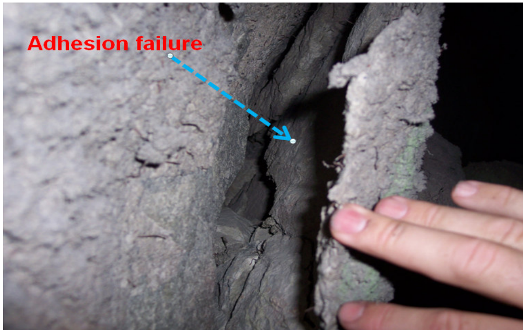
Figure 3.34a Photograph showing adhesion failure of shotcrete on Pillar E at South Deep Mine
