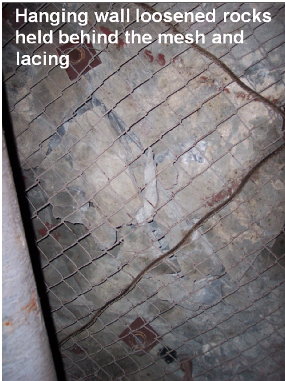
Figure 5.5b Close view of Mponeng Mine Level 109 mesh and lacing section (mesh and lace section in Figure 5.5a) showing loosened rock held back by mesh and lacing support
