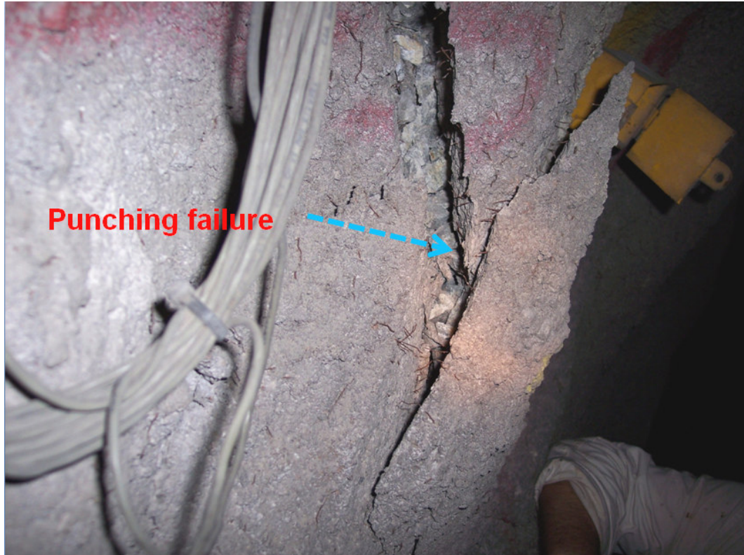
Figure 3.35 Photograph showing punching failure of shotcrete on Pillar D at South Deep Mine
