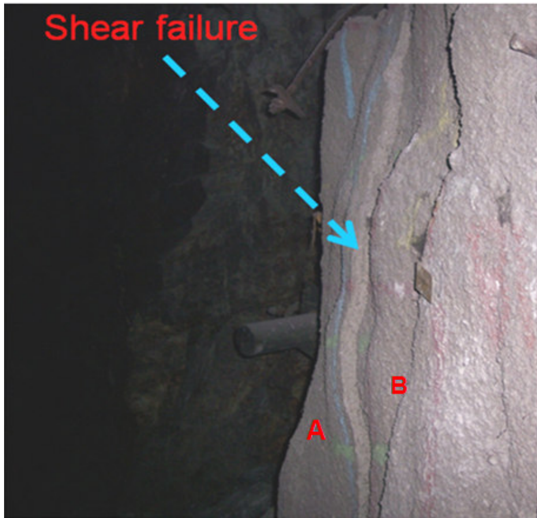
Figure 3.36 Photograph showing shear failure of shotcrete on Pillar B at South Deep Mine
