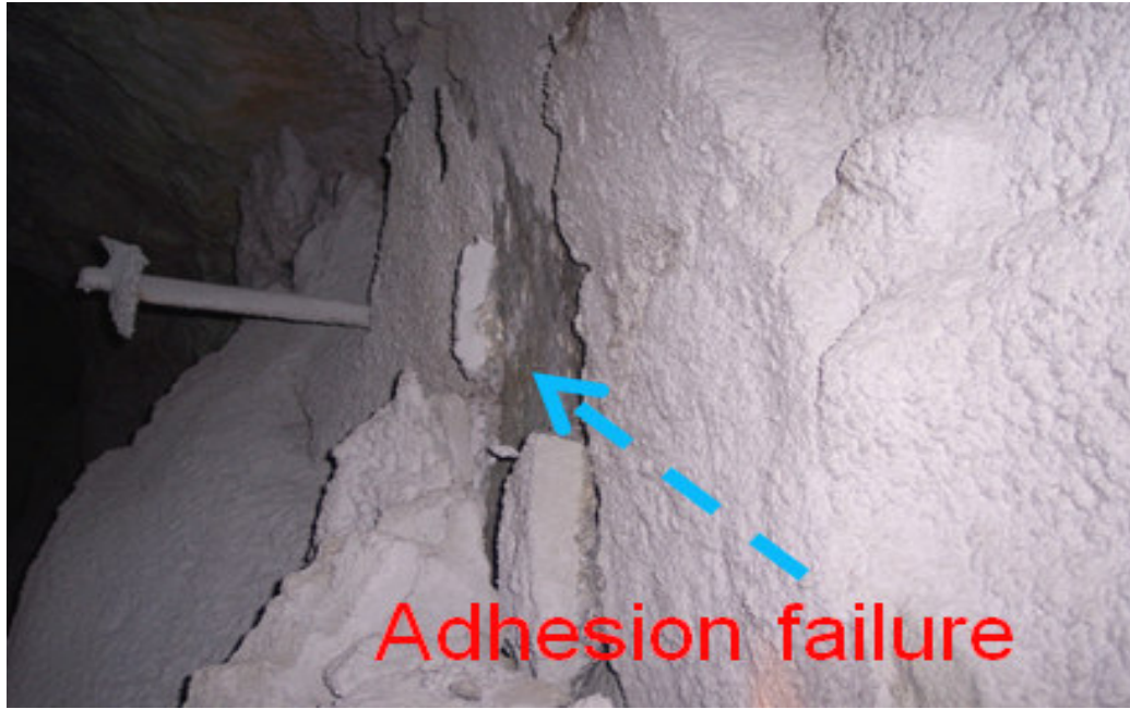
Figure 3.34b Photograph showing adhesion failure between Pillar D and Pillar E at South Deep Mine
