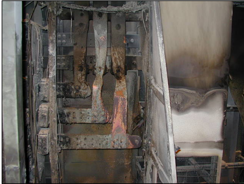
Figure 2.3 Electrical arc flash on a Low Voltage Distribution Board 5
