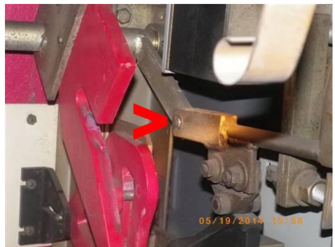
Picture 2: Pin which had broken off
