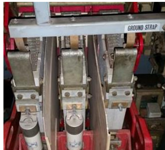
Picture 4 Incorrect maintenance led to the unsafe positioning of the earth strap
