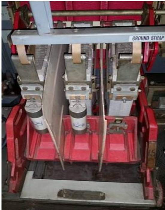
Picture 3 Fused contactor in a racked out and earth position
