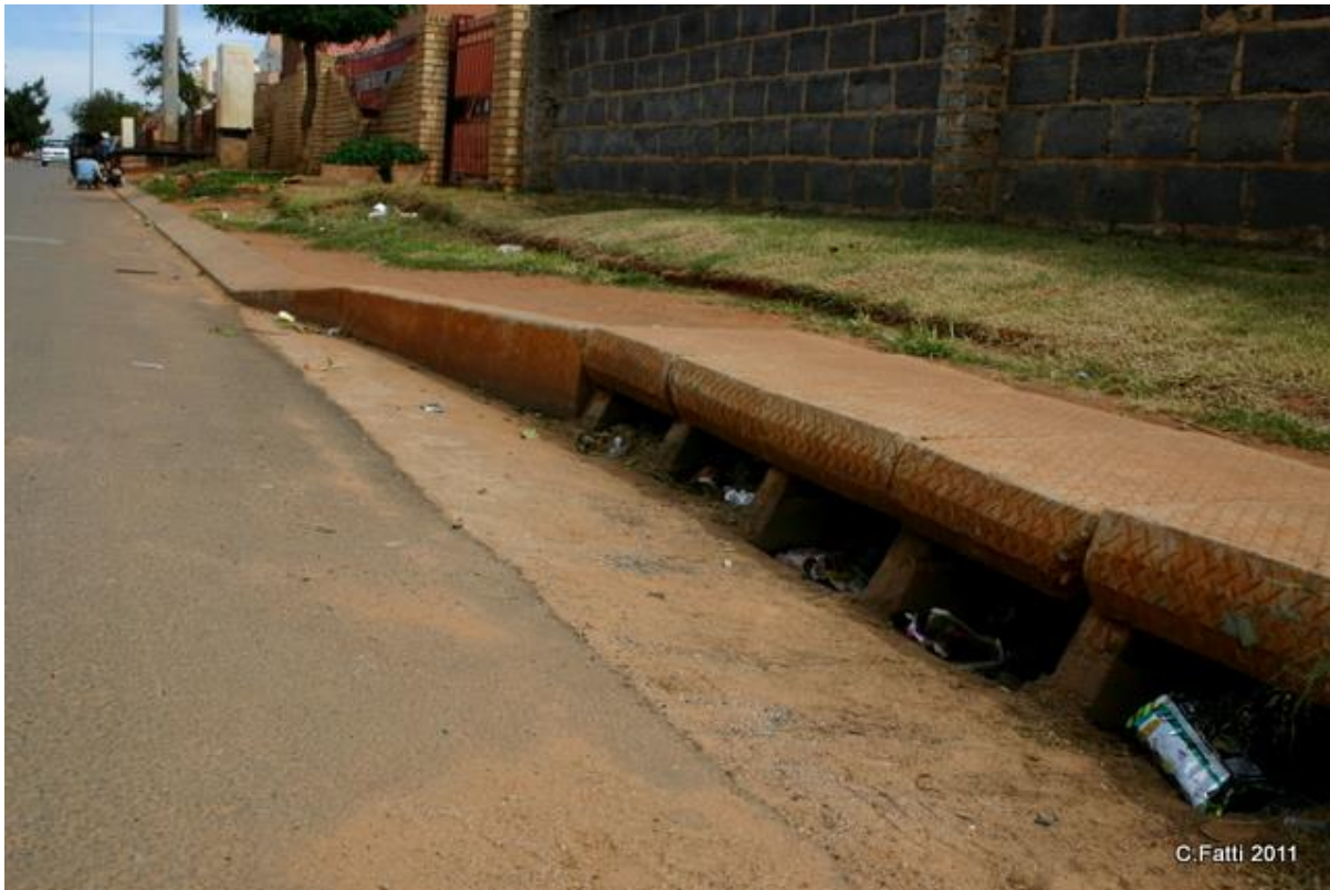
Figure 5.3: Kerb inlet not connected to a stormwater drainage line in Tembisa
