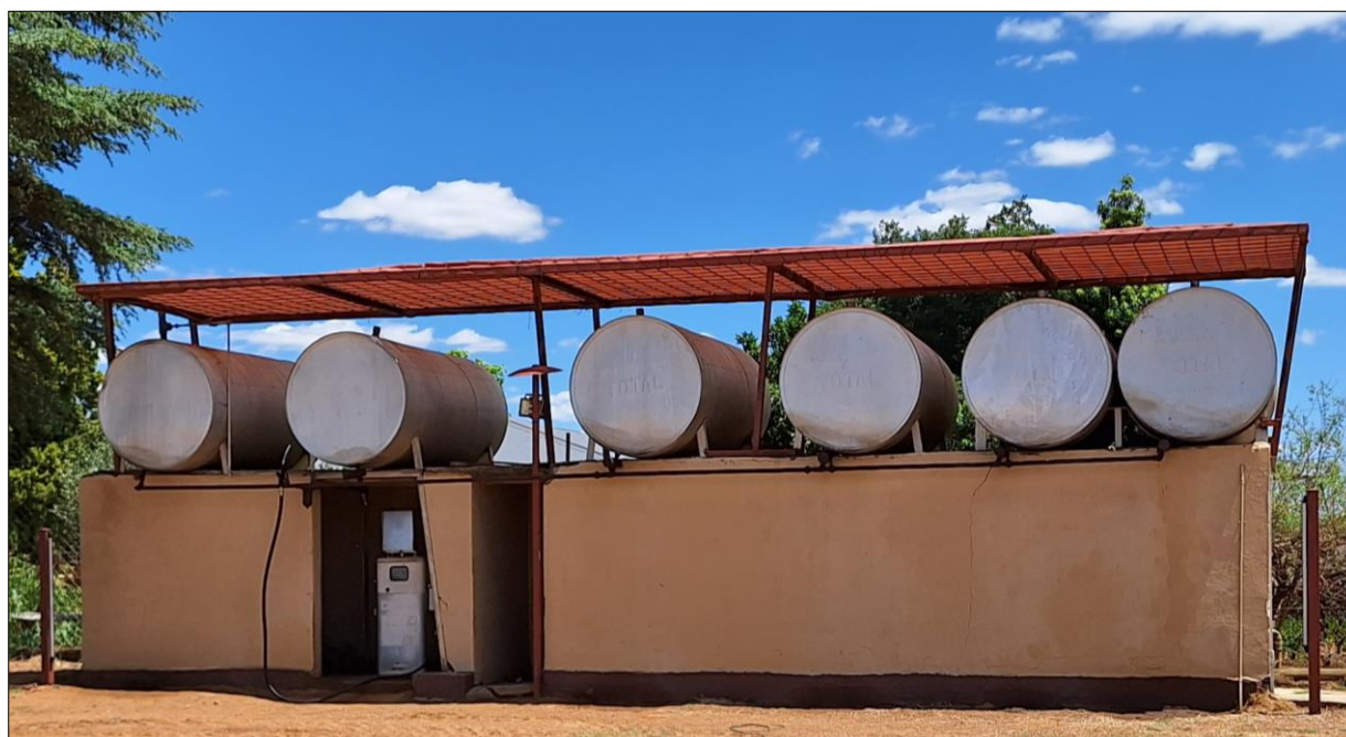
Figure 12: Fuel storage infrastructure. Farm 1.
