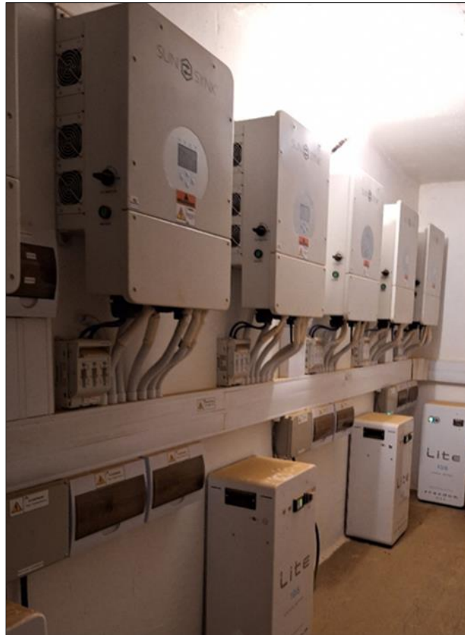
Figure 22: Solar energy invertors. Farm 1.
