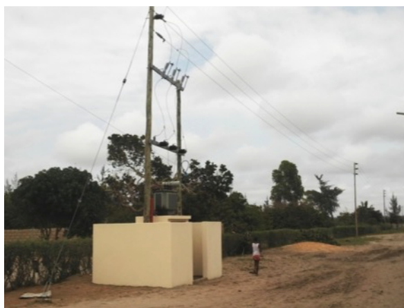
Figure 22 - Electric system and public lighting on the resettlement site. Source: CMM, 2016a.
