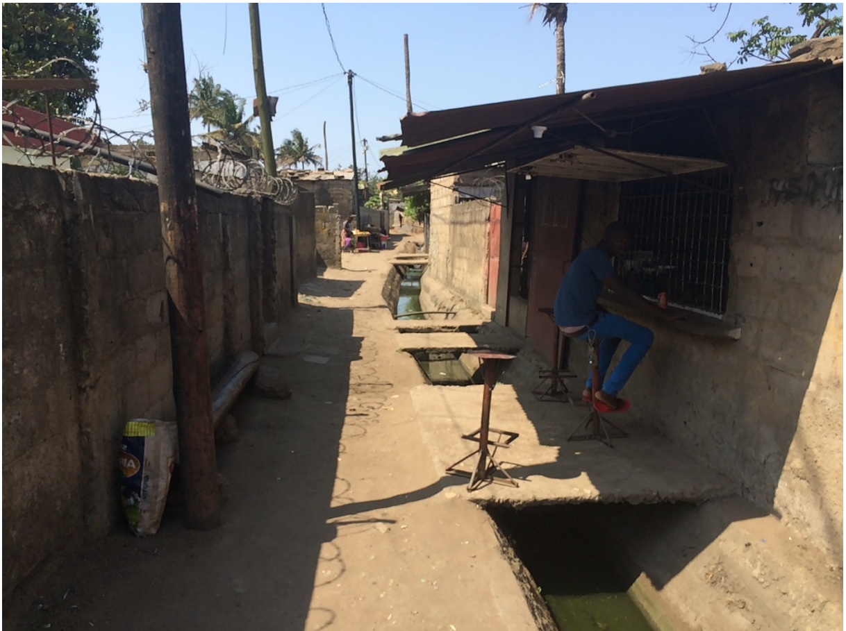
Figure 3: Photo of drainage ditch to be rehabilitated in the neighbourhood of Chamanculo C – Maputo. Source: by author, 2015.
