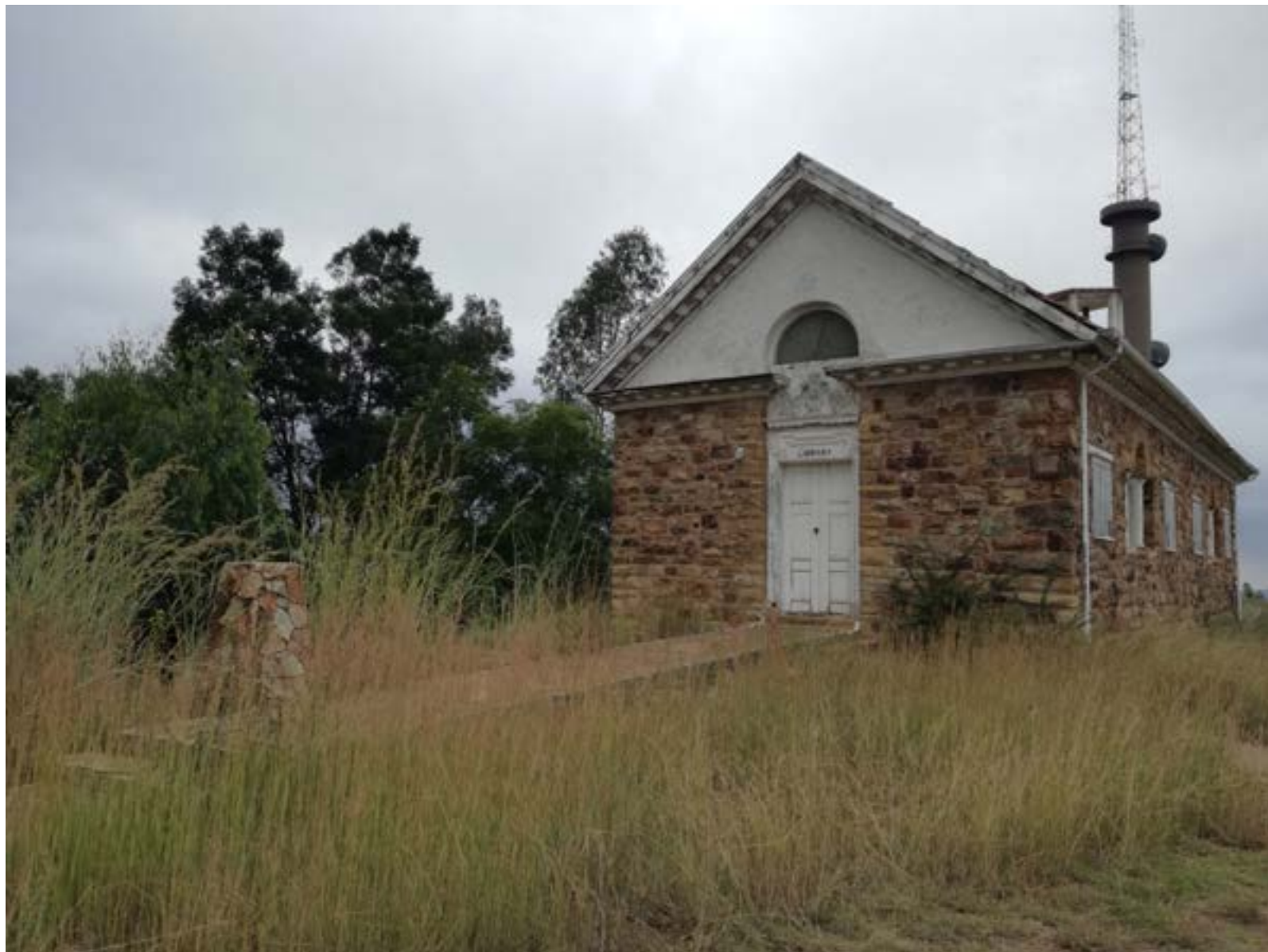
The Herbert Baker Library sits in disrepair. From the outside, it looks relatively untouched. However after closer inspection and looking inside the building one can see that the building has not been taken care of for a long time. It is also made from the previously mentioned quartzite or sandstone and white plaster.
