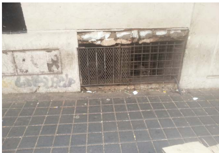
FIGURE 17: Little ventilation exists in this basement
