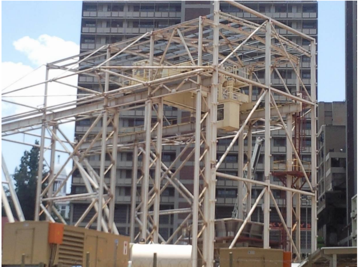
Figure 8:5 A built up column of a crane girder used during Gautrain subway project
