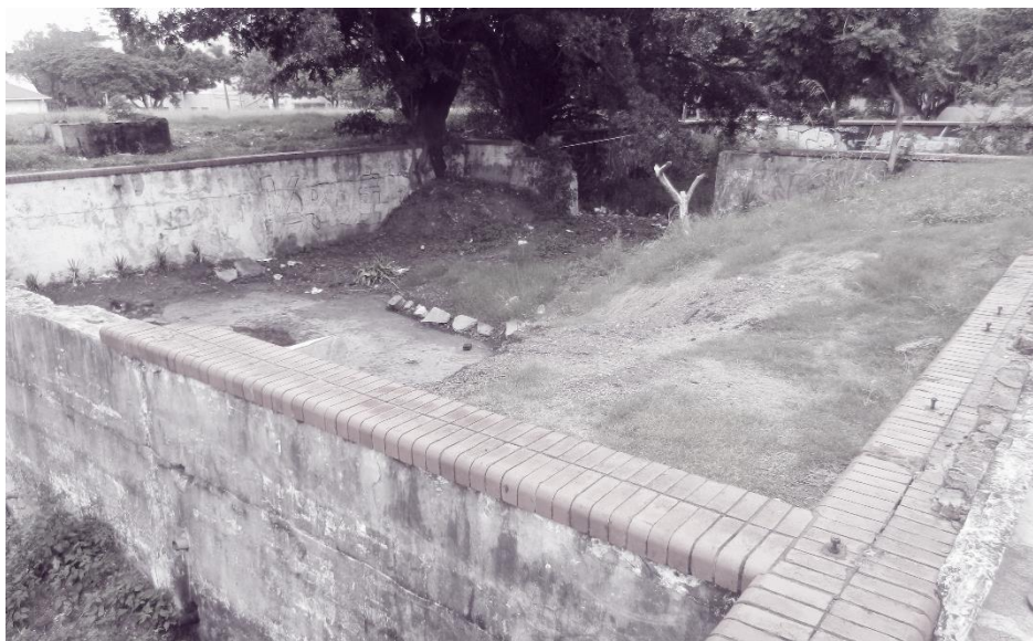
IMAGE 198: Dilapidated Water Treatment Pool (Ndzingani 2020)
