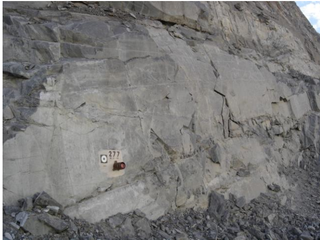
Plate 28 - Protected face prism and target for automated and manual slope stability monitoring
