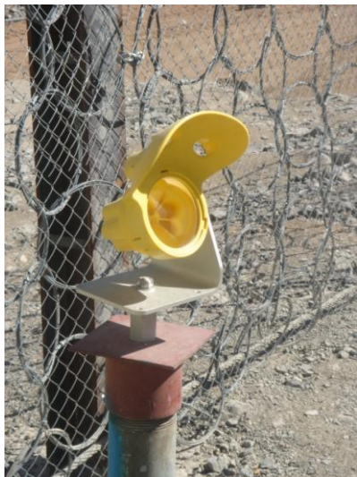
Plate 26 - Crest prism for slope stability monitoring
