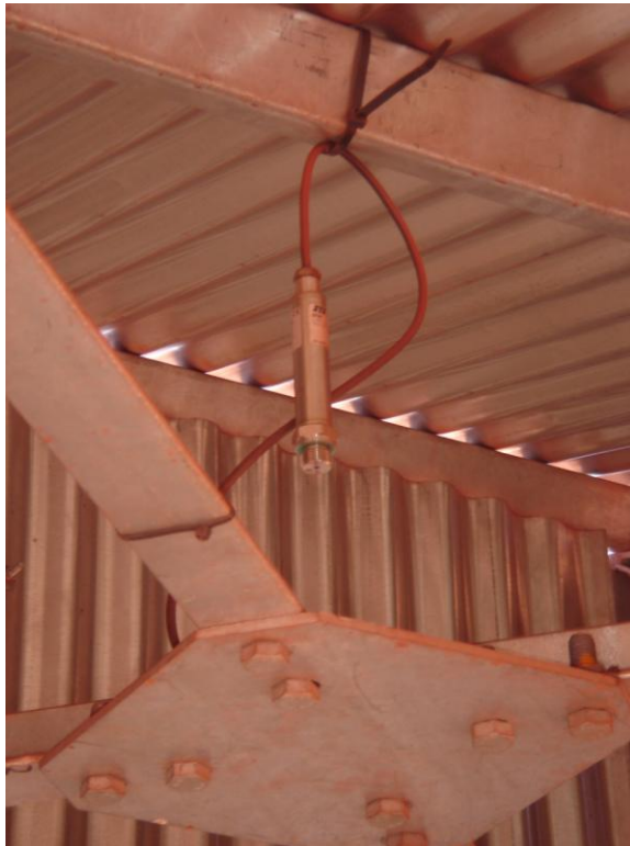
Plate 18 - Meteorological sensor close to the metal roof of the GeoMoS shelter
