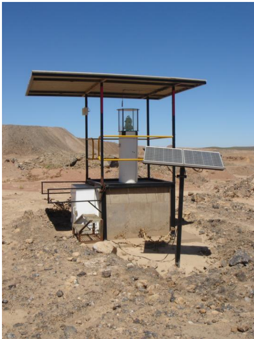
Plate 10 - Slope stability monitoring transfer beacon with protective roof
