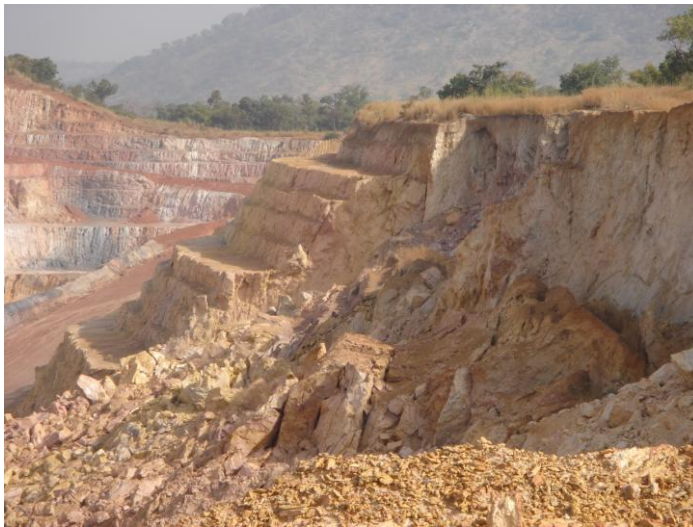
Plate 33 - Composite failure (mix of failure mechanisms - rock mass/circular failure)
