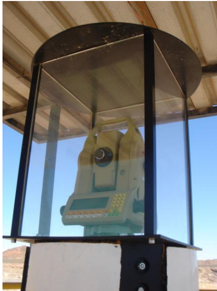
Plate 11 - Slope stability monitoring instrument in protective glass housing
